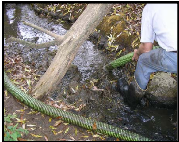
Use a vacuum truck to remove manure from critical sites.
