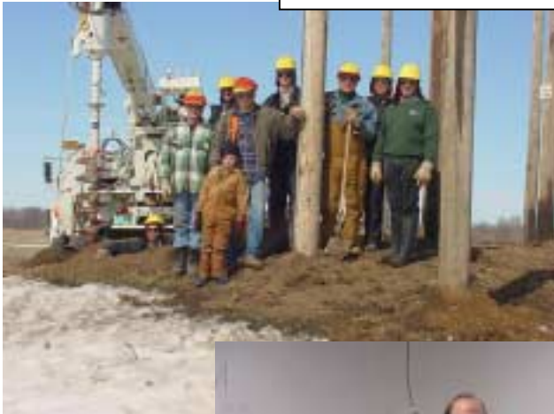
Wisconsin Electric and its employees volunteer 5 hours of service to set utility poles for the support structure for a handicapped accessible wildlife viewing structure.
